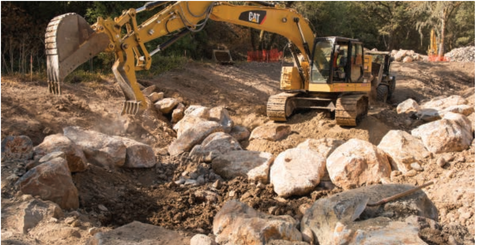
The concrete culvert at Stuart Creek Run that was blocking steelhead from their native spawning grounds further upstream has been removed. Here, contractor Hanford ARC is using an excavator to place boulders in the creekbed to form pools and chutes that will facilitate fish passage. Photo by Lance Kuehne Photography.
